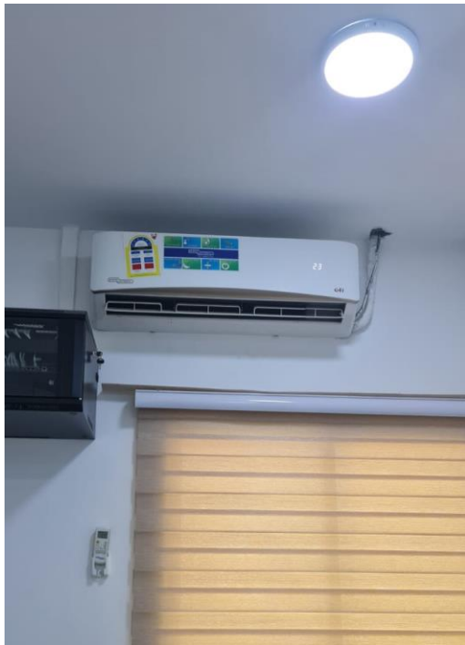
5 Star Energy Saving Air Conditioners in all the offices and buildings, beside insulation.
