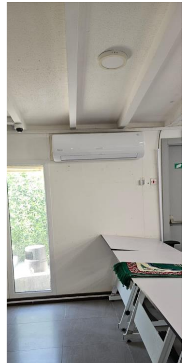
Inverter AC installed in all the classrooms, labs, & library
